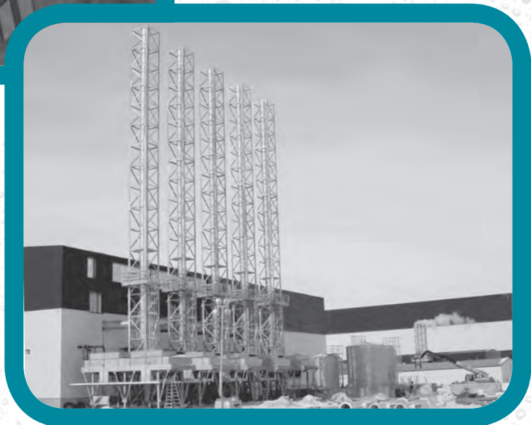
Generator & Fume Exhaust
